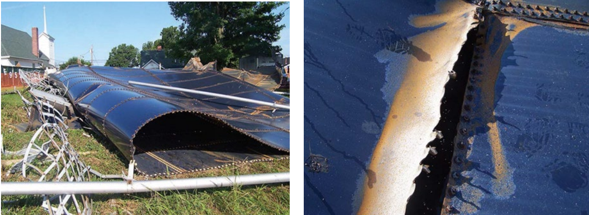
Figure 7. Failed glass-fused bolted steel water tank (Waddy Fire District, Kentucky)
